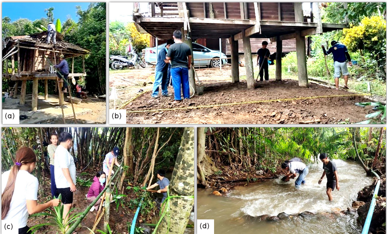
Figure 8 Improving area for the Wisdom bank establishment; (a) Repairing the roof of the Lhong Khao building, (b) Repairing the basement of the Lhong Khao building, (c) Demonstration of planting medicinal plants and (d) Weir construction
